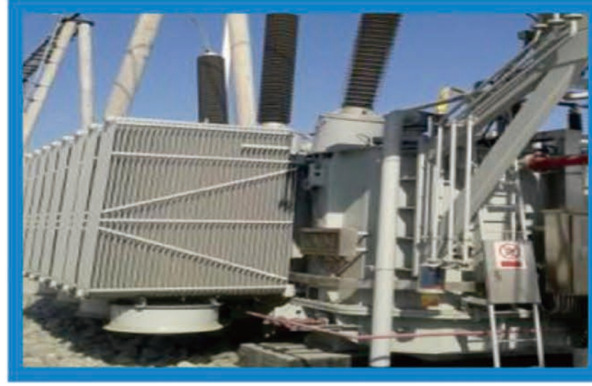
The 252kV RIP transformer bushing operated in the heavily earthquake-prone area of Chile.(Chile)
