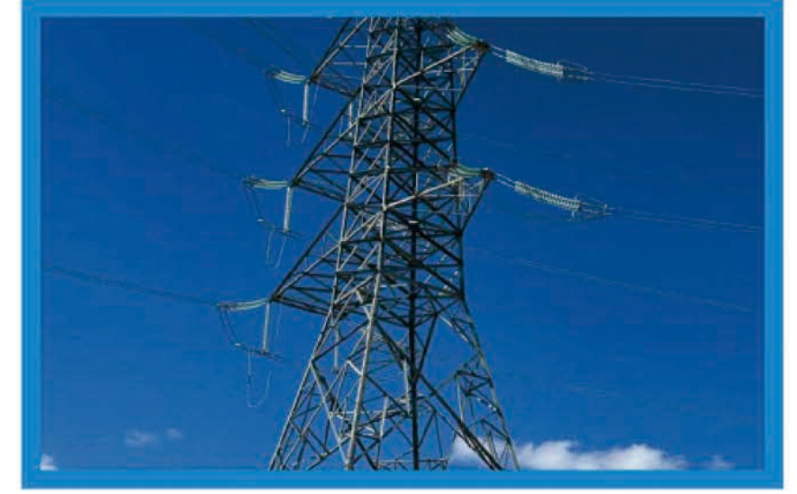
Australia Transgrid 220kV/330kV PEC Project(Australia )
