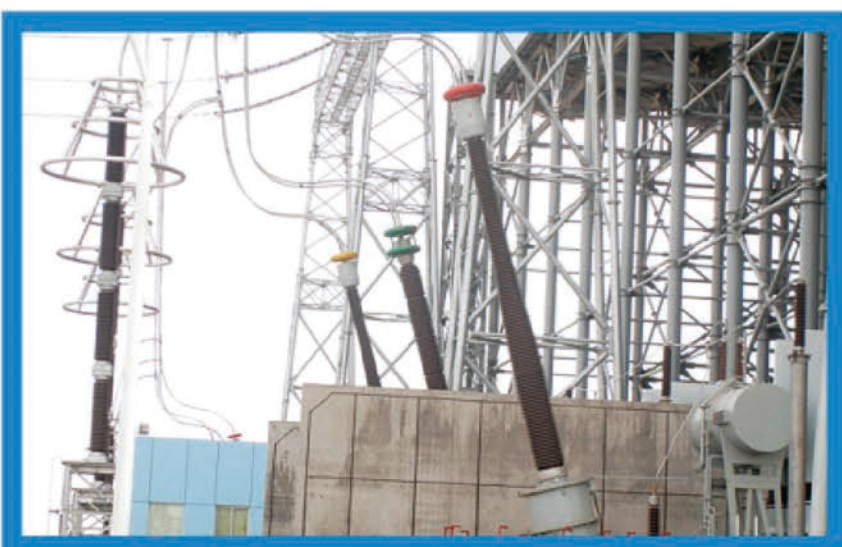
The 800kV OIP transformer bushing is running at the Ningxia Dam.(China)
