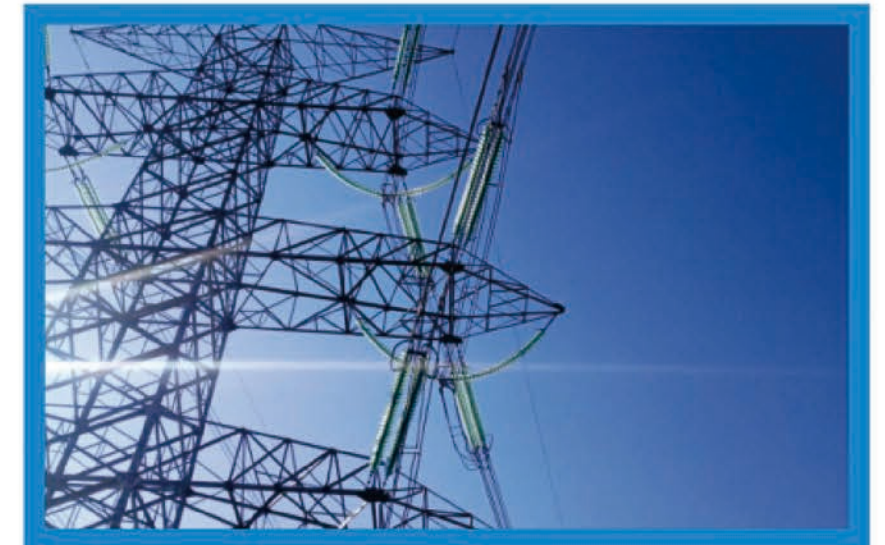
TEIAS 420kV Transmission lines Project.(Turkey)
