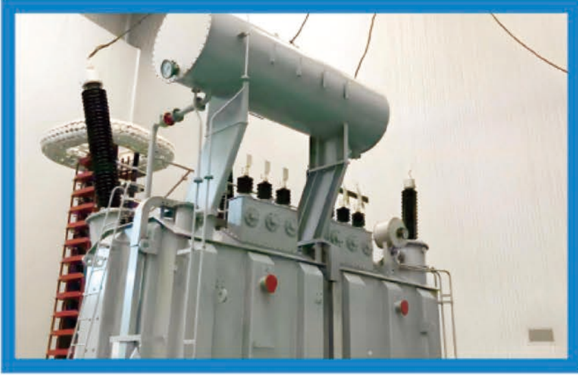
90MVA & 60MVA, 220kV power transform for 900MW liquified natural gas power projects of Ministry of Electricity and Energy of the Government of Myanmar(Myanmar)
