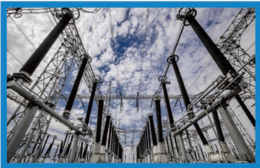
Shanxi Investment Group Xinjiang Wucaiwan North Third Power Plant 750kV Substation(China)
