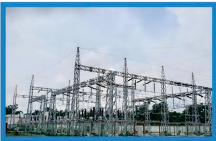
Complete 132kV power substation equipment supply of Sreepur 150±10%MW(BRPL) HFO based power plant project, (Bangladesh)
