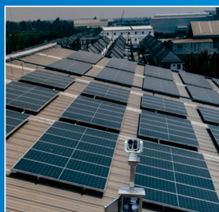
Solar panel on roof
