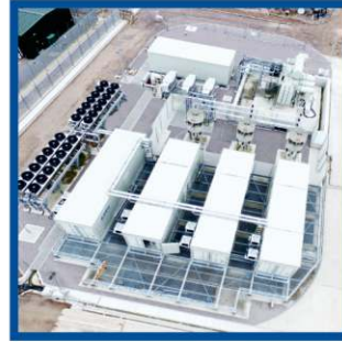
UK Race Bank 2 × ±120MVar STATCOM project
