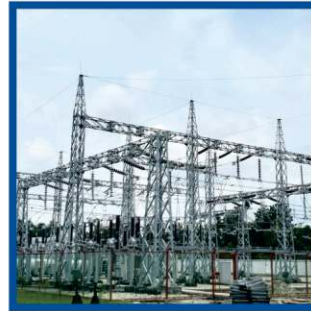
Complete 132kV power substation equipment supply of Sreepur 150±10%MW (BRPL) HFO based power plant project, Bangladesh
