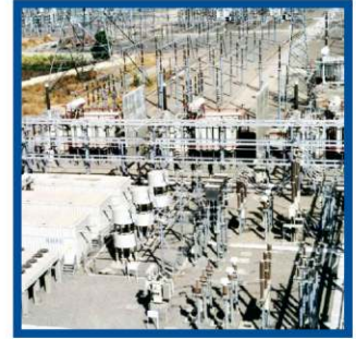
3 sets 400kV, ±300MVar India STATCOM project
